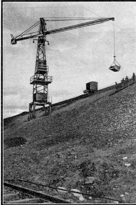
Hammer-head crane engaged in facing head-race canal embankment with broken stone, prior to final covering with concrete slabs
