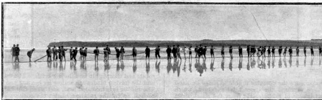
Heavy work on the shores of the Baltic Sea. Hauling ashore the southern end of the telephone cable between Germany and Sweden
