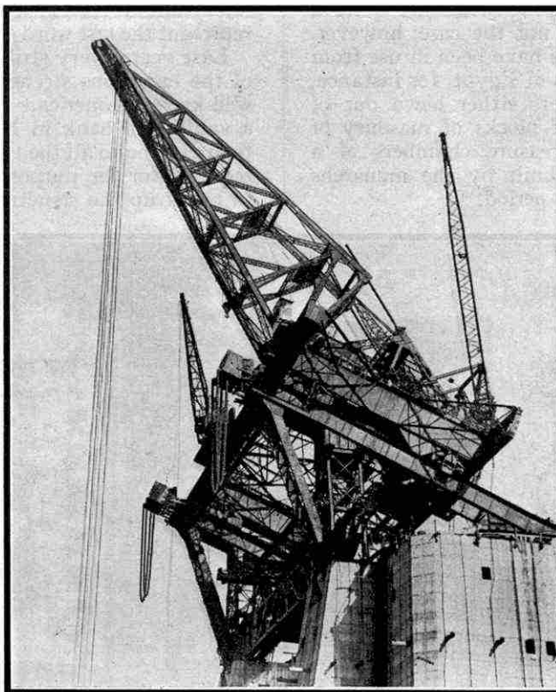
An unusual view from below of one of the "creeper" cranes mounted on the abutment towers of the Sydney Harbour Bridge. (See page 622)
