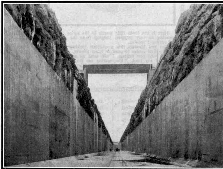
View of the Chippawa-Queenston canal in the rock section. In places the bed of the canal is 143 ft. below the surface of the ground
