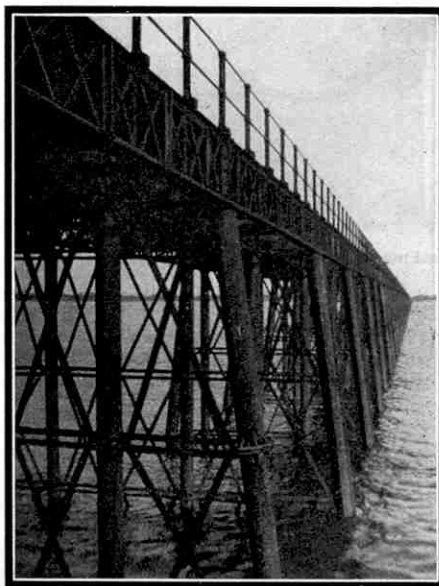
The piers of the Solway Viaduct are of light construction and on one occasion several were broken by ice flocs.
