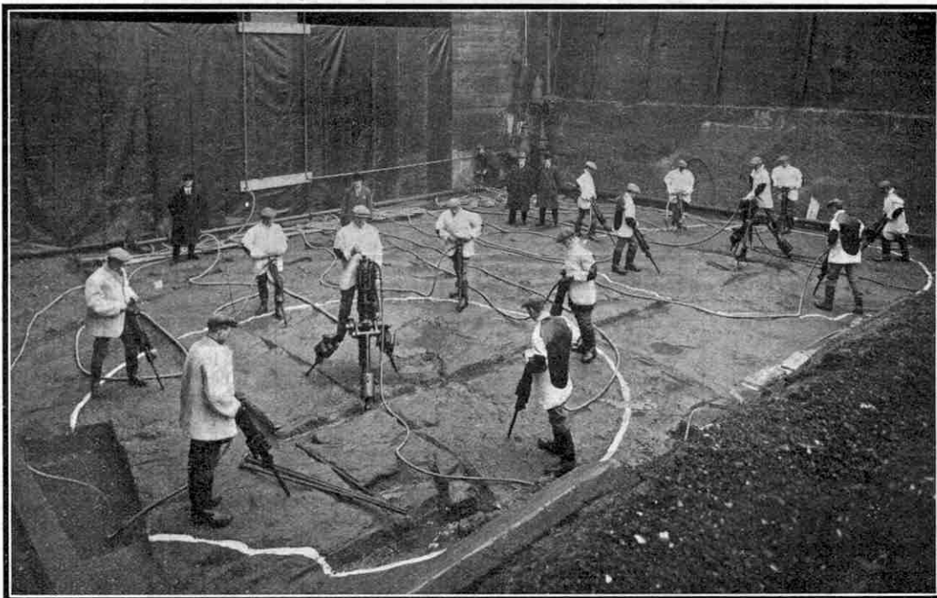
The inauguration of the new Mersey Tunnel operations. Drills ready to commence work on the shafts, which were sunk from the floor of a disused dock. For the illustrations to this article we are indebted to the courtesy of Ingersoll-Rand Company Ltd.
