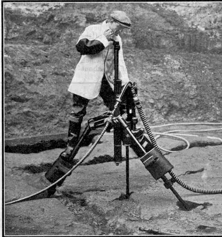
A close-up view of one of the heavier type of compressed air drilling machines used in the new Mersey Tunnel.
