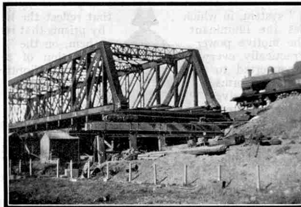
The bridge shown in the upper illustration on this page was erected at the lineside and rolled into position. In the above photograph two of the rollers are clearly visible.
