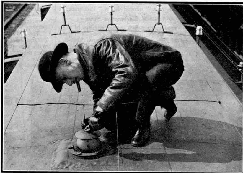
Connecting the transmitting aerial to the lead-in. Mr. J. C. Burkholder, the Chief Engineer of the Canadian National Telegraphs, putting the finishing touches to the wireless telephone apparatus for use on trains, of which he is the designer. On each side of the car are two wires that form part of the receiving aerial.
