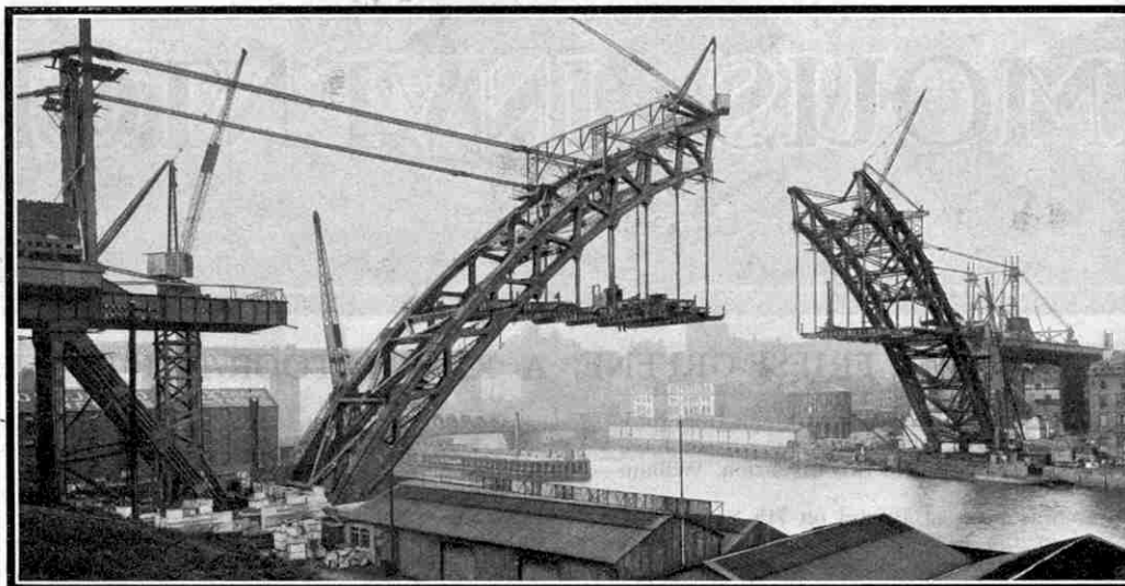
The arch nearing completion. The photograph shows clearly the cables used to support the arch during construction.
