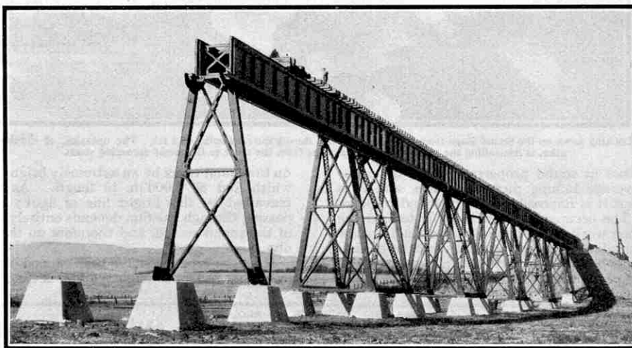
Erecting one of the viaducts of the Martinez-Benicia Bridge that carries the Southern Pacific Railroad across Suisun Bay, America. For this and the other illustrations to this article we are indebted to the courtesy of the S.P.R.
