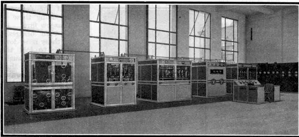
One of the two transmitters at Brookman's Park. On the right is the desk of the engineer in charge, and beyond it may be seen part of the main switchboard.
