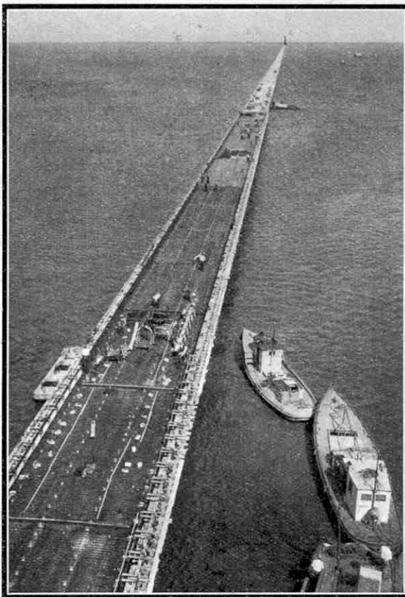
A striking photograph of the James River Bridge taken during construction of the concrete highway. What appears to be a lighthouse in the far distance is actually the lift span seen in the photograph on the opposite page, and is only three-quarters of the distance across. For this and the accompanying photograph we are indebted to the courtesy of the "Scientific American."
