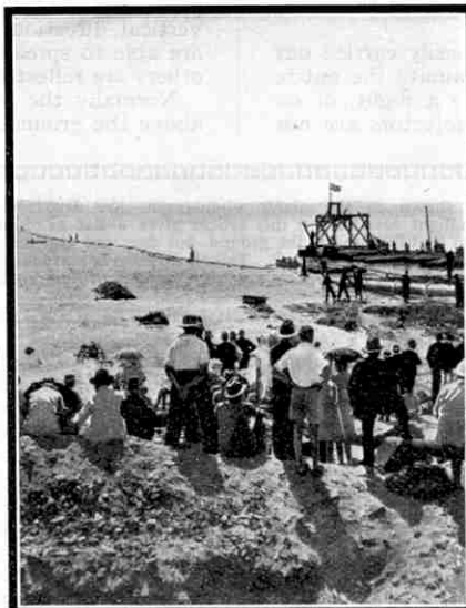
Scene during the launch of the pipe, showing the platform from which the operation was controlled.
