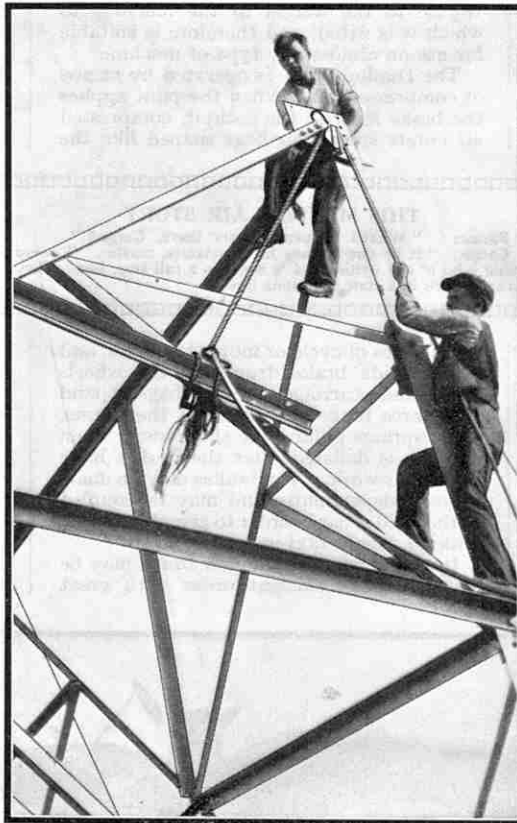
Building one of the pylons on which the overhead transmission wires of the Grid scheme are supported. Photograph by R. S. Jackson, Stacksteads.
