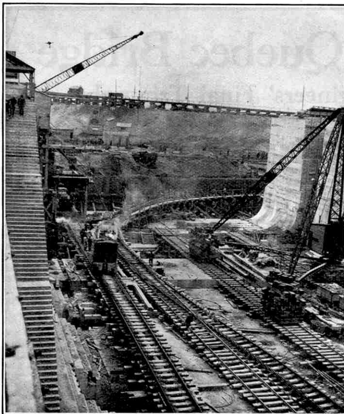
Work in progress on the world's largest dock, which is mentioned on this page. For permission to reproduce this photograph we are indebted to the Southern Railway.
