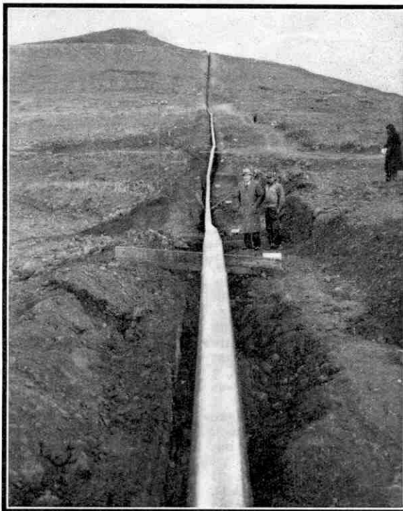
A section of the pipe, treated as described in the article, and ready for lowering.
