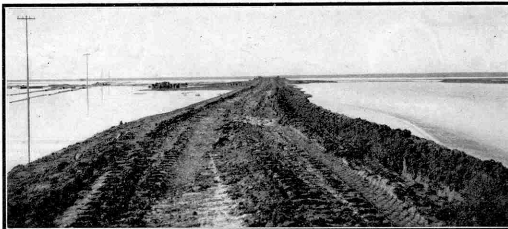
A typical example of the floods that seriously hampered work.
