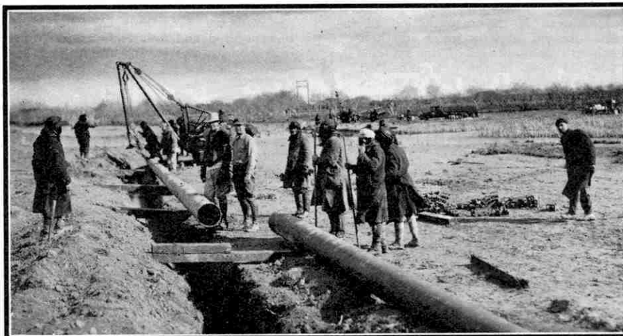
Pipe-laying gang at work near Orontes Crossing, Iraq. For the photographs on this page, and the lower one opposite, we are indebted to the Iraq Petroleum Company.
