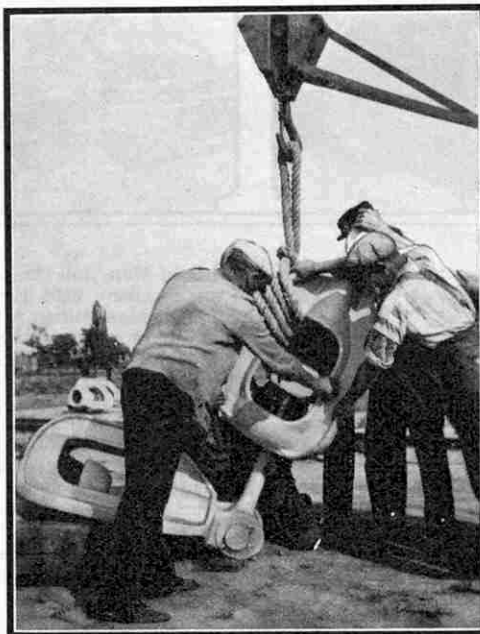
Fitting together the parts of one of the giant insulators in the steel guy ropes that hold the tower in position.
