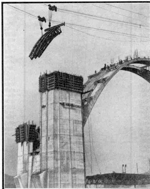
The aerial ropeway being utilised to dismantle the falsework, or centring, after the concrete of the arch rib has set.
