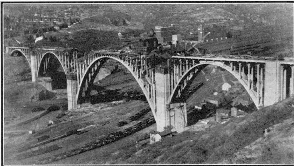
The bridge nearer completion. The arch ribs have been finished and the building up of the concrete columns to carry the roadway and the cantilevered sidewalks is well advanced.
