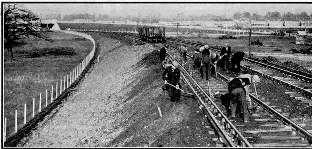
Packing the sleepers up to the correct level before ballasting. The rail is held up by the jacks shown in the illustration to facilitate operations. Photograph reproduced by courtesy of the S.R.
