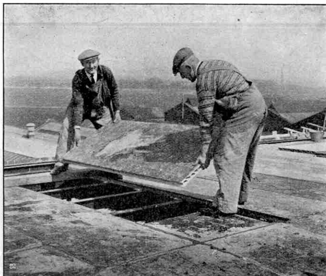
Laying asbestos cement roofing slabs that are built like girders. Photograph by courtesy of Turners Asbestos Cement Co., Manchester.
