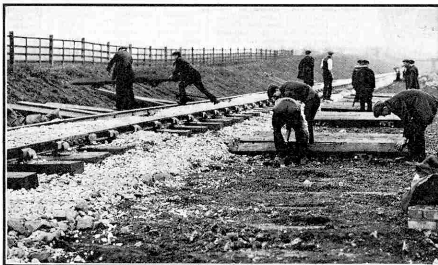
Removing the sleepers of the temporary track to make way for the main line material. The track alongside is already laid, and the ballast has been tipped ready for spreading. Photograph reproduced by courtesy of the L.M.S.R.
