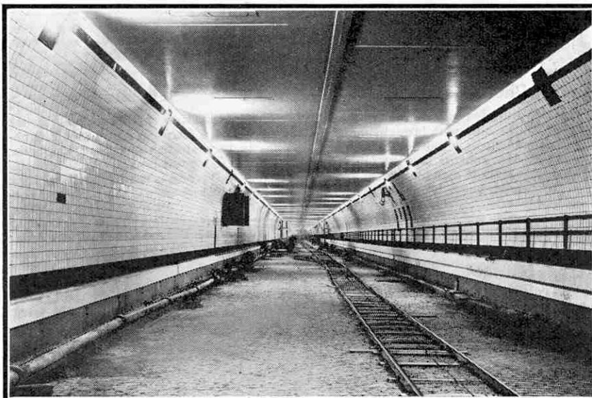
The vehicular tunnel under the River Scheldt at Antwerp, nearly completed, but before the roadway was laid down. The illustrations to this article are published by courtesy of Société des Pieux Franki.
