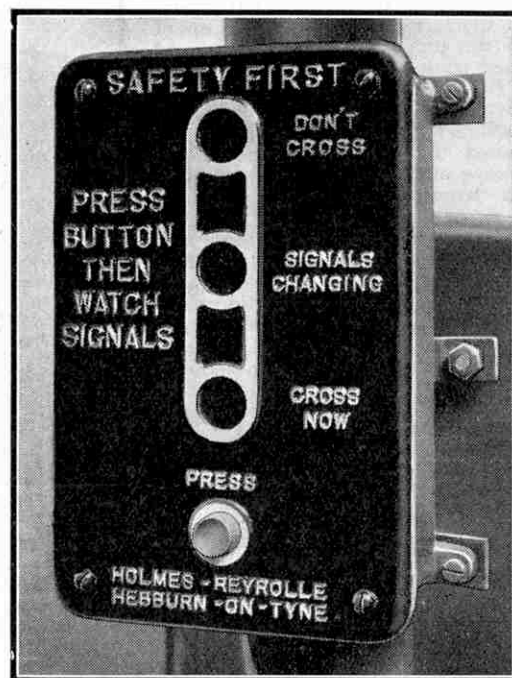
One of the pedestrian push-button control boxes.
