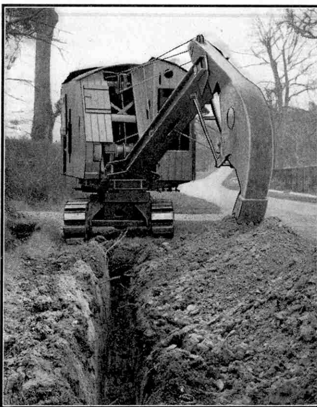
The Priestman "Cub" excavator with "Teredo" attachment for cutting narrow trenches. Photograph by courtesy of Priestman Brothers Ltd.
