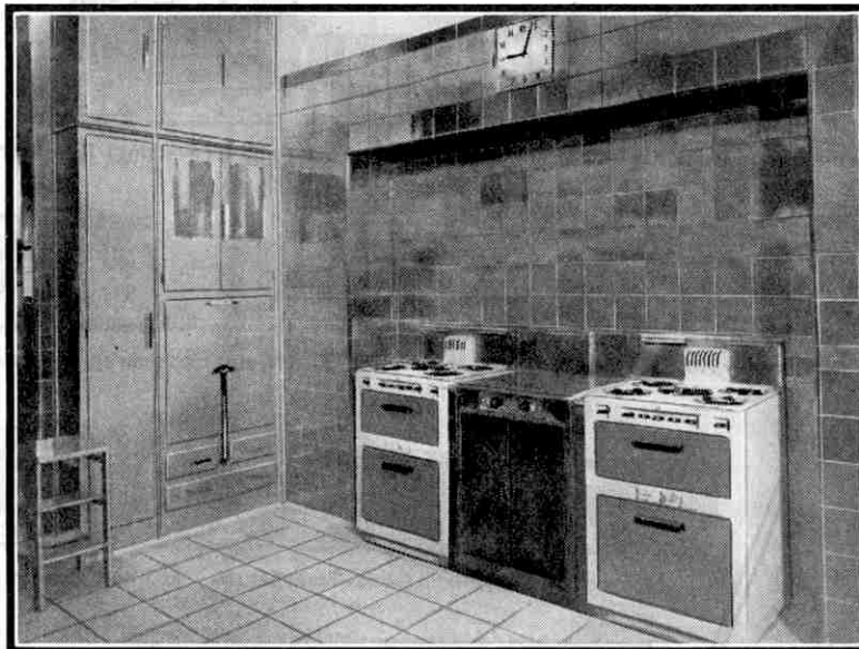
A modern gas cooker of streamline form. This is a replica of the cooker installed in the King's House. Photograph by courtesy of the British Commercial Gas Association.
