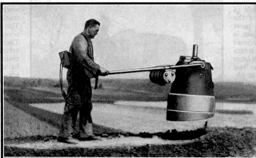
The frog rammer in action. It weighs half a ton and jumps into the air as it delivers its blows. Photograph by courtesy of C. H. Johnson and Sons Ltd., Manchester.
