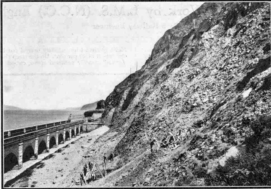
Workmen clearing the site for the viaduct foundations. The L.M.S.R. railway viaduct is shown on the left.
