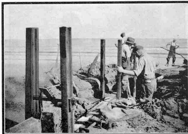
Fixing groynes formed of old rails and timbering on the seashore in front of Dawlish Station. Photograph by H. M. Madgwick, Worthing.
