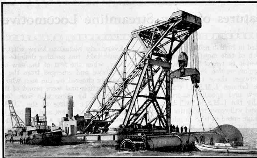
The "Gironde" lowering a 290-ton reinforced concrete pile before bringing it into a vertical position with its wider end resting on the ocean bed.
