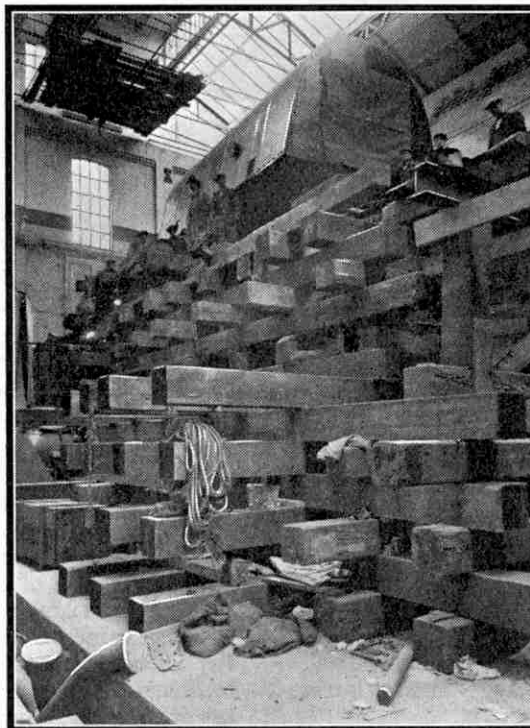
An 82-ton stator for an electric generator being lifted into position at the Brimsdown Power Station. The illustration shows the large amount of packing required to support the stator while it was being lifted. For our illustration we are indebted to the Metropolitan-Vickers Electrical Co. Ltd.
