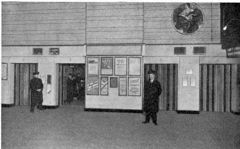
General view of the four new lifts. They are electrically-driven and are controlled automatically. A mechanical voice gives warning when the gates are about to close.
