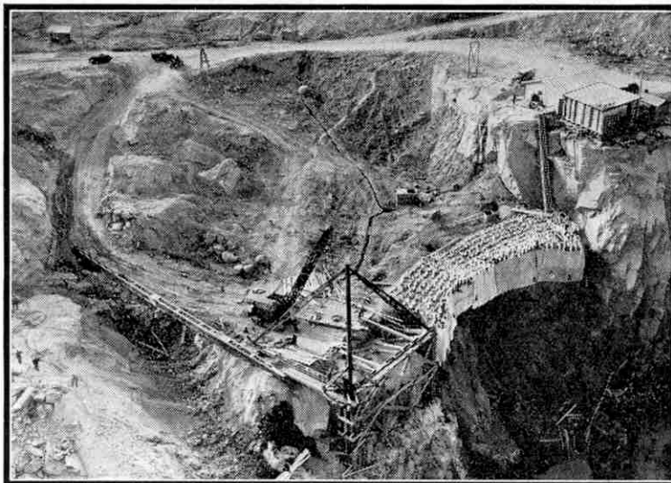
Landslides that threatened an excavation were prevented by the frozen earth dam shown above. Pipes through which frozen brine was circulated can be seen projecting above the dam.
