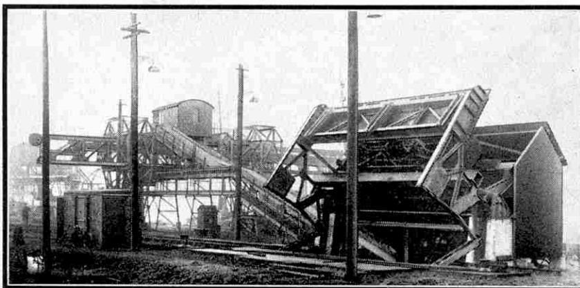
One of the six new coaling plants recently installed at Fleetwood docks for bunkering trawlers. In the foreground is the wagon tippler, and beyond it is the travelling gantry that extends outwards from the quay. For our illustration we are indebted to Mitchell Engineering Ltd., London.
