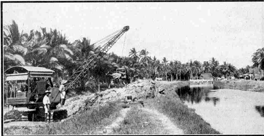
A Priestman "Cub" dragline excavator raising the banks of an irrigation canal in northern Malaya. The illustrations to this article are reproduced by courtesy of Priestman Bros. Ltd.
