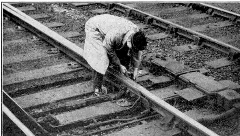
A "Safety-First" operation; a pointsman clipping the switch blades of facing points in position at Paddington. This practice was followed during the period of emergency working, when points had to be hand-operated, after the fire that occurred in the arrival signal box last November. Photograph by W. S. Garth, Luton.
