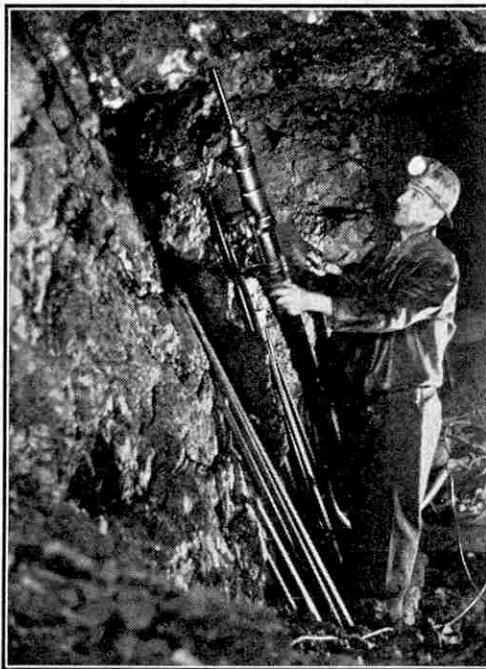
Drilling in progress in the pitchblende mines at LaBine Point in readiness for blasting.
