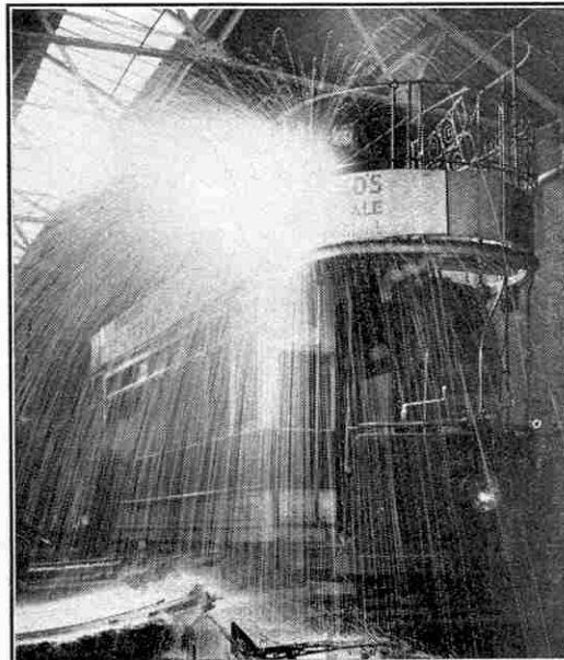
Another way of dealing with old tramcars. The one shown is being cut up by means of the oxy-acetylene blowpipe.
