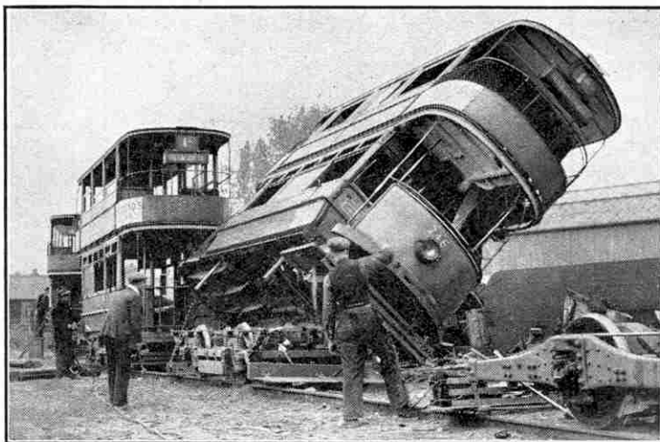
Breaking up old tramcars. After pulling the bodies over on their sides they were set alight to burn out unwanted woodwork. The illustrations to this article are reproduced by courtesy of George Cohen, Sons and Co. Ltd., London.
