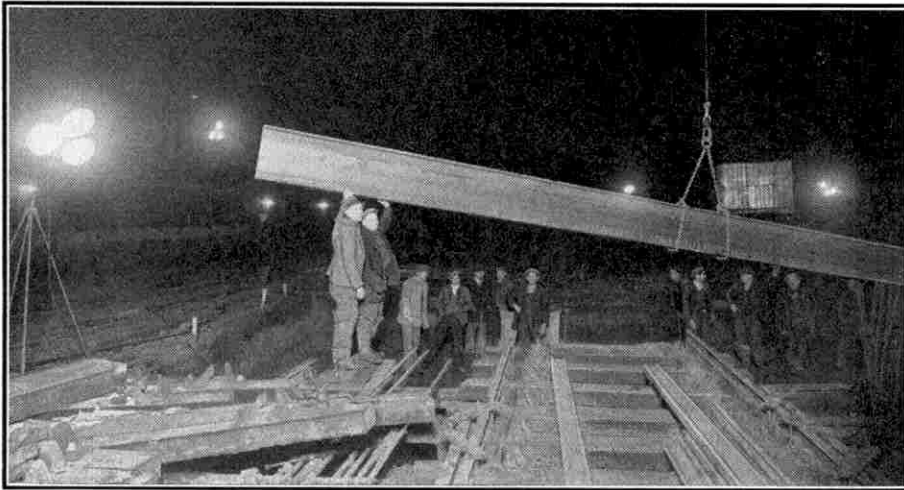
Night work. One of the cross girders for underpinning the L.N.E.R. line being put into position.
