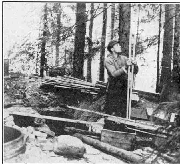
Finnish soldiers building a shelter in the Karelian forests. The picture is taken outside the main line of defence.
