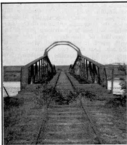
Approach to the swing bridge over the River Blyth. Note the blackberry bush on the track!
