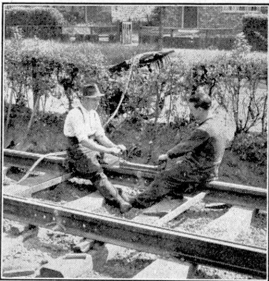
Filing a welded rail joint on the Townsend Avenue Light Railway, Liverpool. Photograph by courtesy of the City Engineer, Liverpool.
