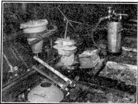
Pre-heating rail ends in a mould before pouring the thermit steel required to join them. This illustration and those on the opposite page show thermit welding of rails on the Glasgow Corporation subway and are reproduced by courtesy of Murex Ltd.
