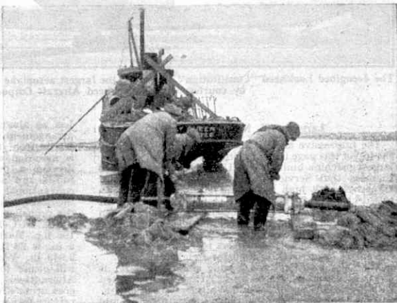
Duddon Estuary: Power Cable joint being buried. The illustrations to this article are by courtesy of Siemens Brothers and Co. Ltd.
