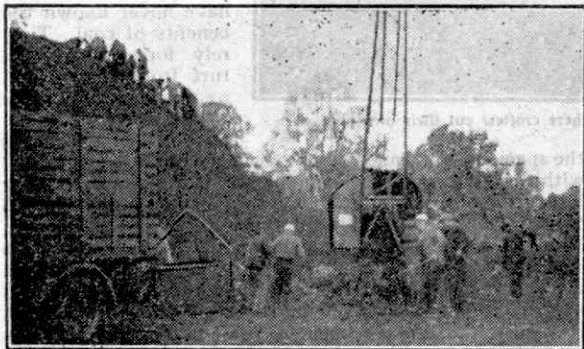
Stacking by crane in progress in Phoenix Park. Peat shovelled into containers is hoisted to the top of the stack.
