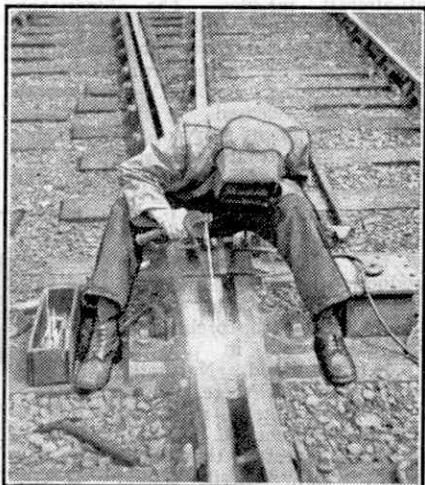
The welder building up a wing rail. Note the spare welding rods in the box.
