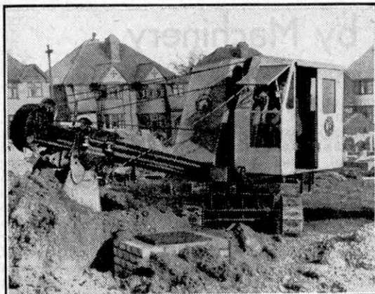
"Wolf" excavator, weighing 9½ tons, with a Skimmer attachment, levelling a road site on a housing estate.
