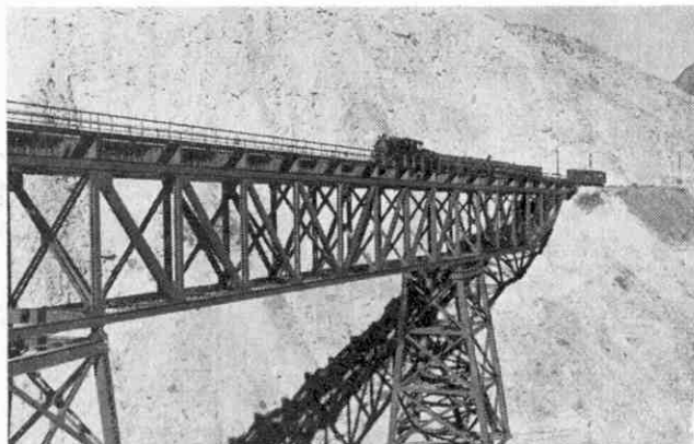
The Carrion Bridge, with a span of 717 ft., is named after the famous Peruvian doctor, Daniel A. Carrion, who sacrificed his life in an attempt to discover the cause of verruga fever. It is the third bridge erected on the site.
