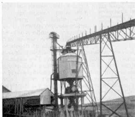
The plant for weighing, batching and mixing concrete. The main conveyor for materials enters at the top, the cement entering through the tube running up the left of the tower.
