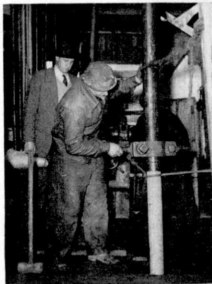
A drilling rod being adjusted inside the 54-ft. high drilling rig on the top deck of the tower.
