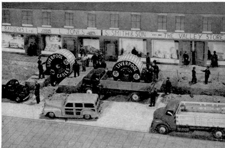
Handle with care! Cable drums being unloaded ready for use in a busy cable laying scene.
