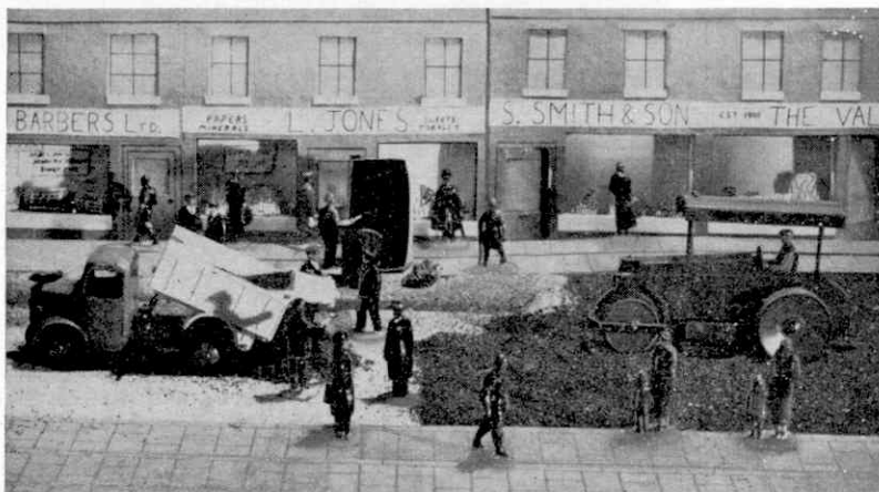
In this view the cable has been laid and an Aveling Barford Diesel Roller is at work on a new road surface over the excavations.
