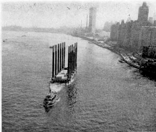
A floating platform used for drilling in the Atlantic being towed up the East River, New York. This picture shows very plainly the steel tubes that were driven into the sea bed.
