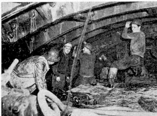
A daily force of 200 men, usually referred to as "sand hogs," worked in compressed air when driving the third tube of the Lincoln Tunnel under the Hudson River.
