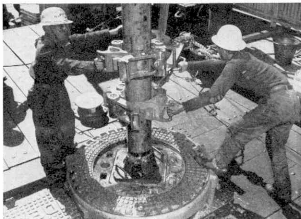
Local Arab trainees making the first joint on the drill collar during operations with the first drilling platform. The drill collar is the heavy alloy steel pipe that gives the weight needed at the bottom of the drilling string.
