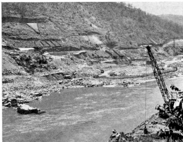
The site on which the Kariba Dam will stand across the Zambesi River, looking downstream. This picture shows early work in progress. The illustrations to this article are reproduced by courtesy of the Federal Information Department, Southern Rhodesia.
