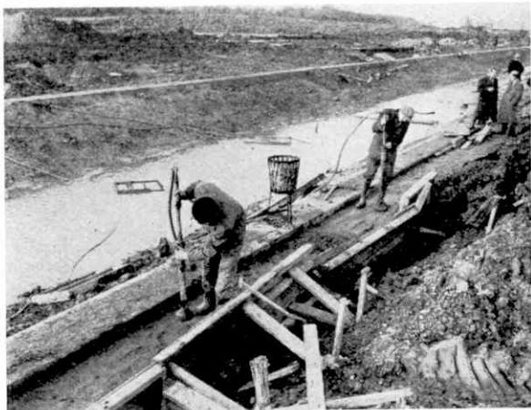
The new canal section has concrete walls on each side, with puddled clay behind them. Here workmen are seen pressing the clay down.
