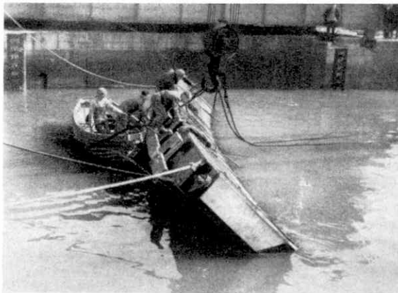
A leaf of the gates of one of the Docks of the Dover Harbour Board being re-positioned.
