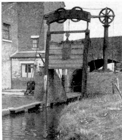
Guillotine gates on the stop lock at Kings Norton.
