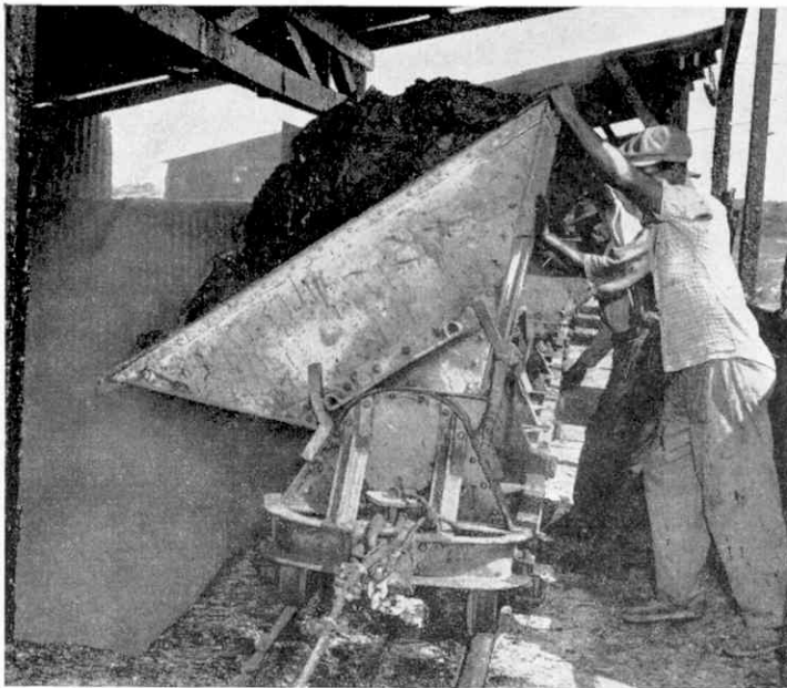
Asphalt being tipped into huge tanks where it is refined by having the water and gas driven off by a simple dehydration process.
