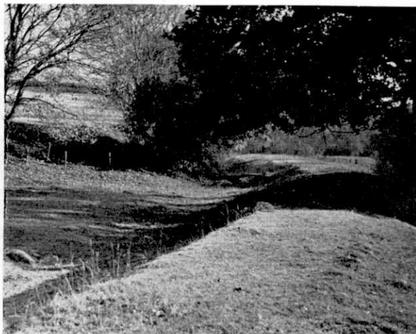
A typical section of the dried-up canal bed. In the middle distance is a small brick dam, once used to keep water in the abandoned canal for use as a fishery.
