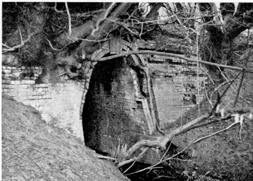
The south-east portal of the old Sousnet Tunnel, near Mamble. The roof has fallen in not far inside, and it would be a dangerous venture to try to explore it. Photographs by the author.
